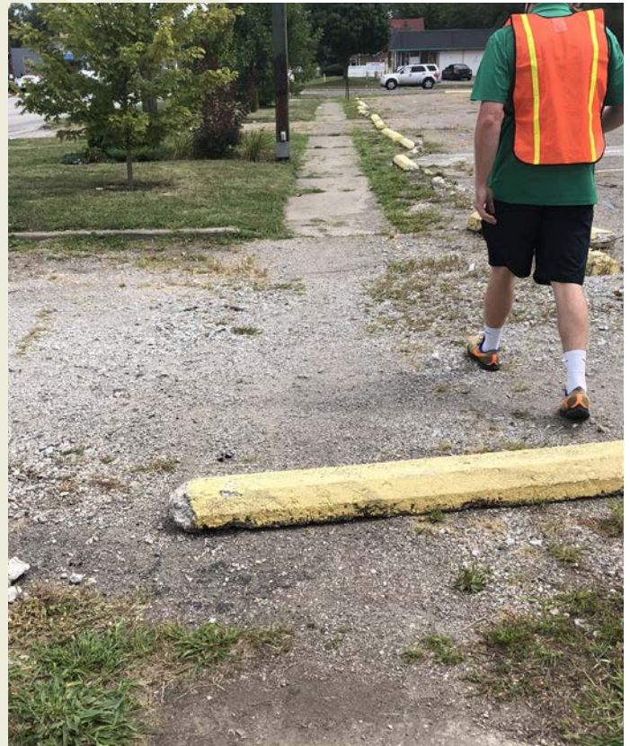
On the south side of E. 38th St. near its intersection with Orchard Ave., a curb stop creates a tripping hazard and blocks passage for persons using mobility devices. As of 2023, this site and much of the 38th St. corridor is undergoing extensive infrastructure enhancements as part of IndyGo's Purple Line bus rapid transit project.
