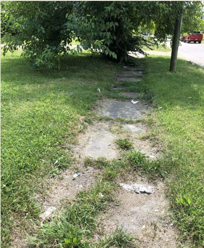
This segment of sidewalk on LaSalle St. near its intersection with E. 25th St. is in poor condition with overgrowth, inhibiting safe and comfortable access to pedestrians, especially persons using a mobility device.
