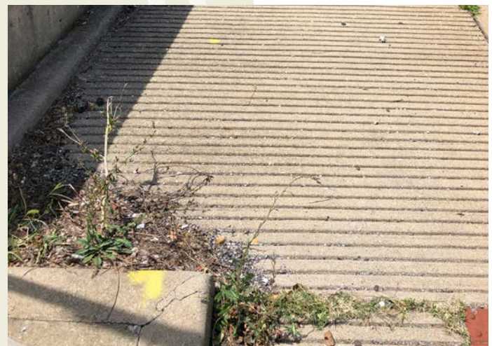
Overgrowth and debris observed at the intersection of W. 29th St. and N. Illinois St. This sidewalk can be challenging and dangerous for pedestrians with no or low vision and persons using wheelchairs or mobility devices due to the placement of utility poles (Crash Zone 9).
