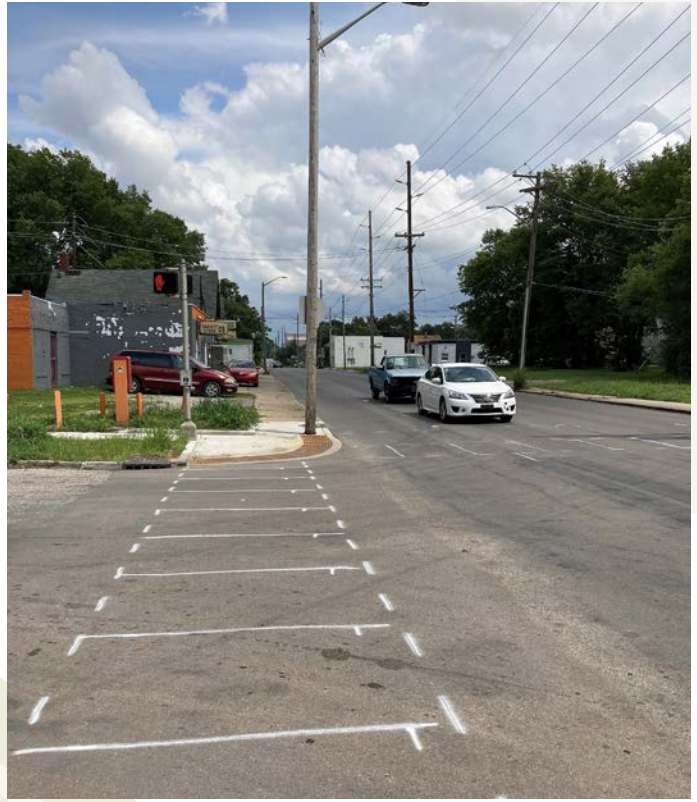
Temporary markings visible at the intersection of W. 10th St. and N. Pershing Ave. in anticipation of new high-visibility crosswalks. A recent repaving of the corridor necessitated new roadway markings in August 2020. A newly installed ADA-compliant curb ramp with detectable warning system is visible at the northeastern corner.
