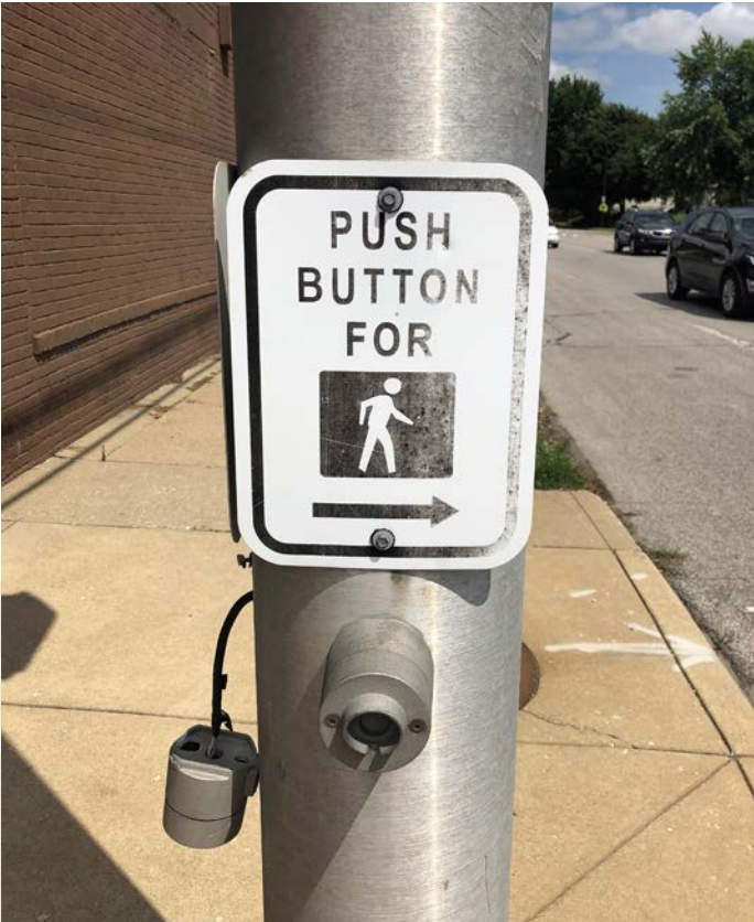
A damaged pedestrian push button dangles from a post at the intersection of W. Michigan St. and Belmont Ave., looking east. The issue was documented and submitted via RequestInly and has since been fixed.
