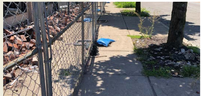
A temporary chain link fence creates a potential barrier for people with disabilities or persons who are blind or low vision. Intersection of Boulevard Pl. and W. 40th St. (Crash Zone 4).
