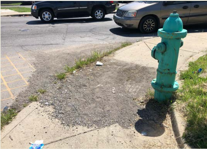
Gravel, dirt, debris, weeds, and weathered crosswalks create an unsafe walking environment, especially for those with no or low vision. Intersection of W. 29th St. and Dr. Martin Luther King Jr. St. (Crash Zone 8).
