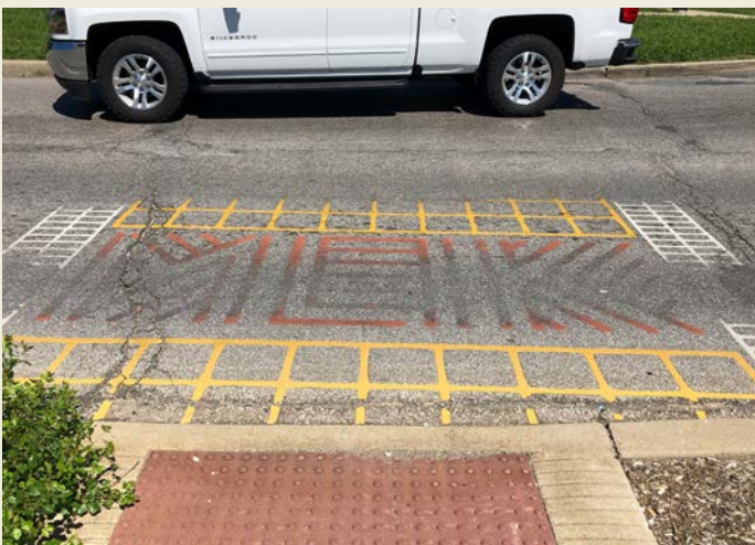
With proper maintenance, duratherm crosswalks, like this one on Dr. Martin Luther King Jr. St., can add to a neighborhood's unique character. Unfortunately, this duratherm crosswalk has weathered and isn't visible to motorists (Crash Zone 8).
