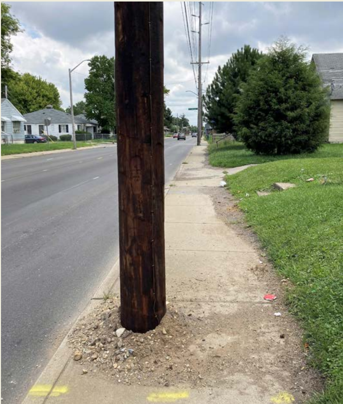
A utility pole recently installed in the sidewalk near the intersection of W. 10th St. and N. Centennial St. Utility poles in sidewalks are common along the W. 10th St. corridor. Accumulated debris, also present throughout the corridor, poses a tripping hazard to pedestrians.
