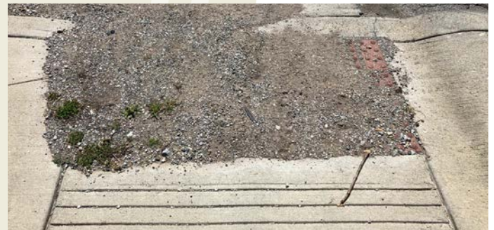
During Walk Audits, participants make note of potential challenges for pedestrians. Though up to design and safety standards, many curb ramps in this area of Indianapolis suffer from neglect, collecting gravel, dirt, and debris that can make it difficult for pedestrians with mobility and vision challenges.
