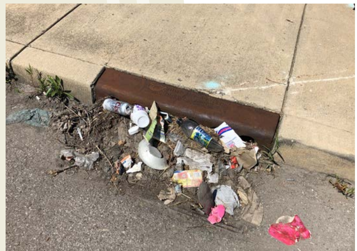
Litter that accumulates in storm drains, like this one in Crash Zone 8, can cause flooding of both the roadway and nearby crosswalks. Keeping storm drains clear also ensures our waterways are clean and healthy.
